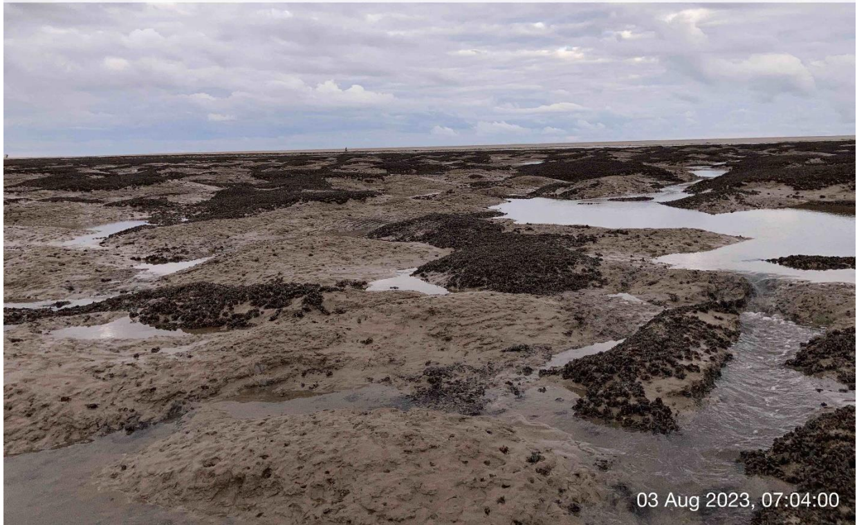
Figure 15. Evidence of scour on Perch Scar 03-08-2023.
